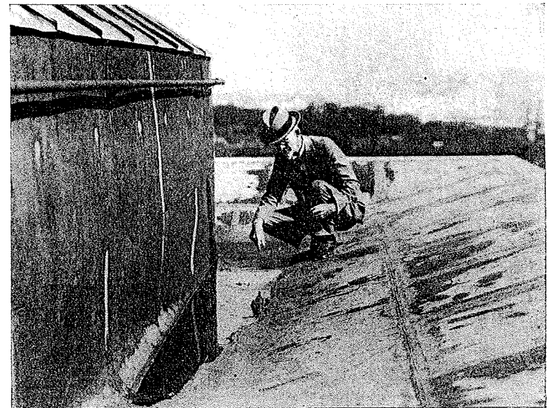
Figure 3 Corner in wide gutter, showing a pool of water
